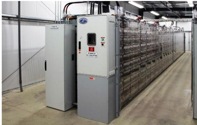
Figure 2.26. Three strings of batteries installed. Source: (DOE, 2015)
