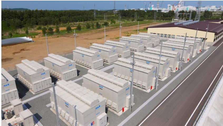
Figure 2.32. 17 sets of 2 MW NaS batteries. Source: (Kawakami et al., 2010)
