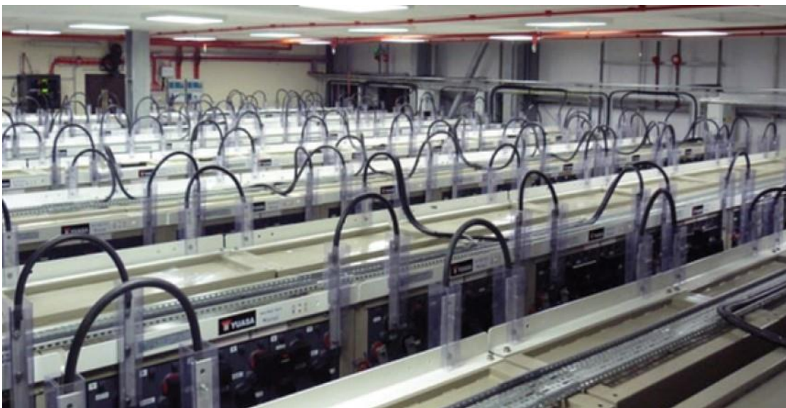
Figure 2.25. Battery room at Lerwick Power Station. Source: (GS Battery Inc., 2016)
