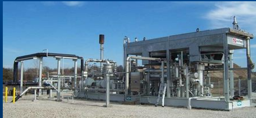
Blower, Flare and Treatment System
