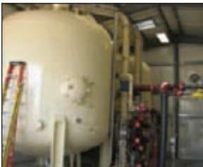
Activated Alumina Vessels.
