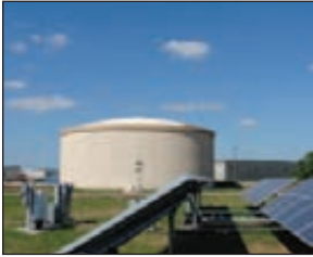
Solar Array at the San Benito Water Treatment Plant.
