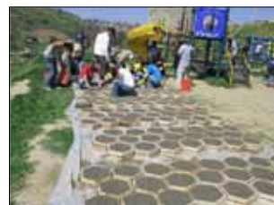
Volunteers arrange pavers that allow water to percolate through the pavement and channel runoff.
