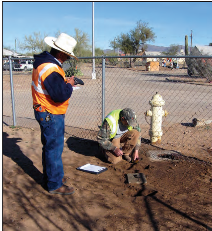
Utility workers in Sells, Arizona, plot the location of a water main, a practice known as "potholing."
