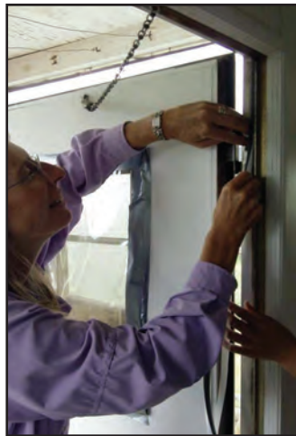
A Viva Verde contractor installs weather stripping to the door frame of a southern New Mexico home.
